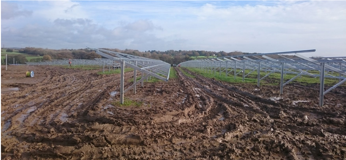
Inserts 36 and 37: Winter Installation (2015) and Operational Site (2022)
